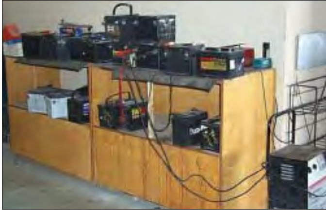
Indoor used battery recharge area, batteries stored or recharged on wood shelving, over an impervious surface, recharge areas should be well ventilated (wood shelving does not corrode).
