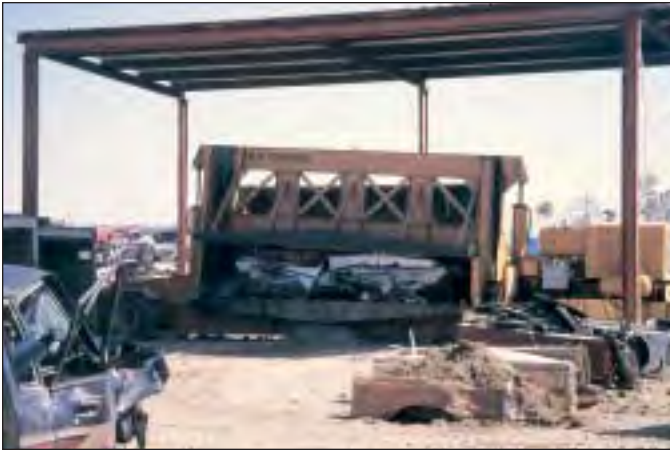
Crusher used to crush properly drained and stripped cars; crusher situated beneath a shed on an impervious surface.
